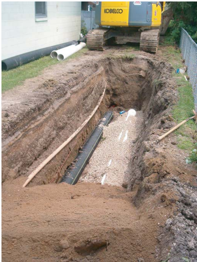
Gravity Sewer Line
